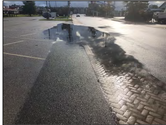
Figure 13: Standing water on Gordon Stinnett Ave.
