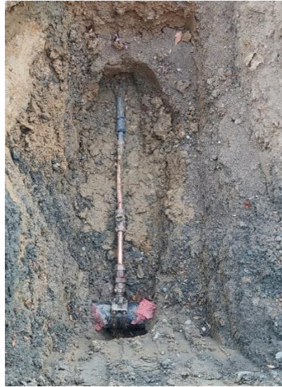
Picture 7 Eyewash/Emergency Shower Tie In
