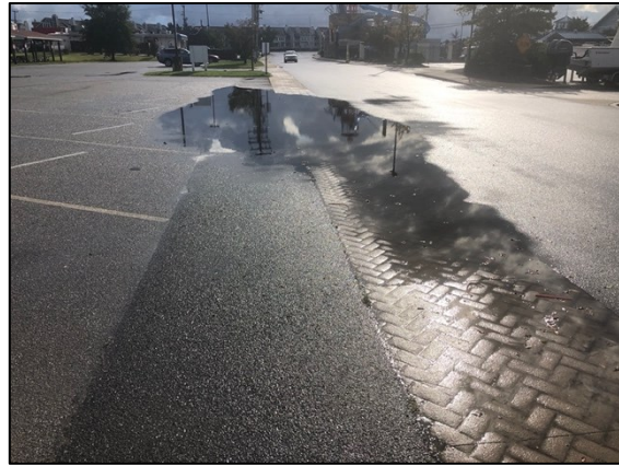
Figure 13: Standing water on Gordon Stinnett Ave.
