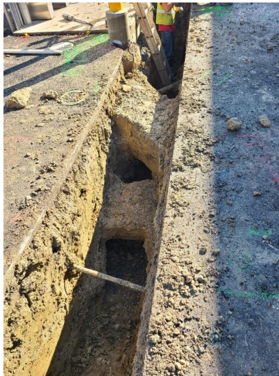
Picture 4 Duct Banks and Piping
