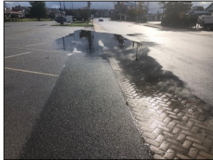
Figure 1243: Standing water on Gordon Stinnett Ave.
