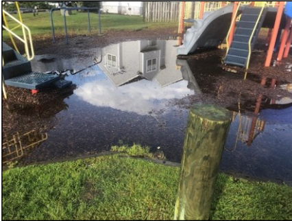
Figure 1142: Standing Water at the Tot Lot at Kellam's.
