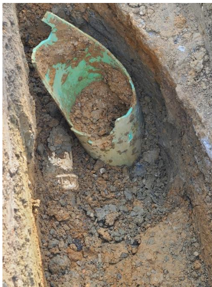
Picture 2 Sump pipe and Compression Coupling
