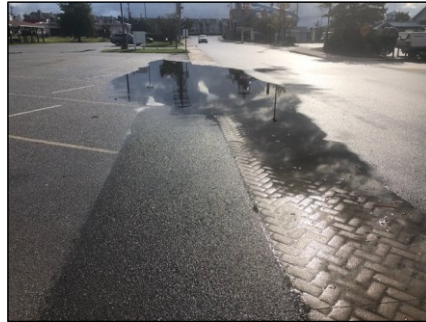
Figure 13: Standing water on Gordon Stinnett Ave.
