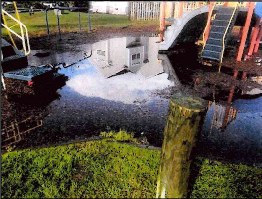
Figure 3: Standing Water at the Tot Lot at Kellam's.
