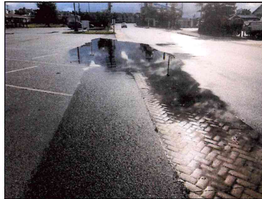
Figure 4: Standing water on Gordon Stinnett Ave.
